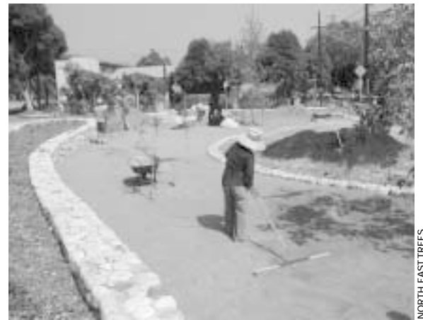
North East Trees crews prep for the installation of a decomposed granite path in Blake Park, one of many neighborhood parks springing up along the Los Angeles River.
